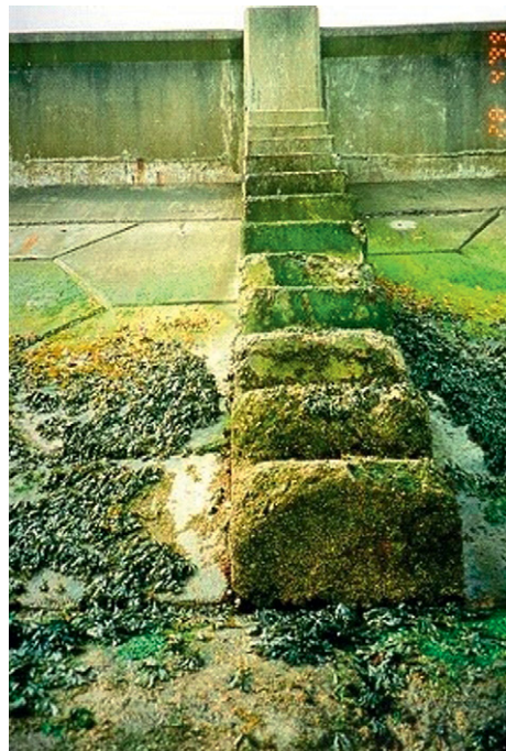
Figure 6 External sulfate attack.
