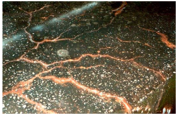
Figure 5 Typical crack pattern of ASR.
