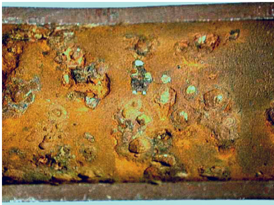
Figure 10 Tuberculation corrosion of steel; corrosion is localized beneath rust protuberances (known as tubercles).
