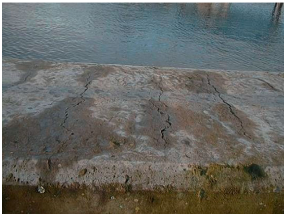
Figure 1 Plastic settlement cracking.
