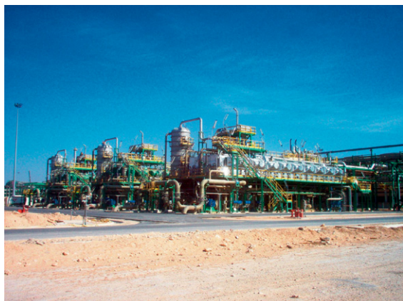
Figure 51 An example of a desalination plant, Melitha.
