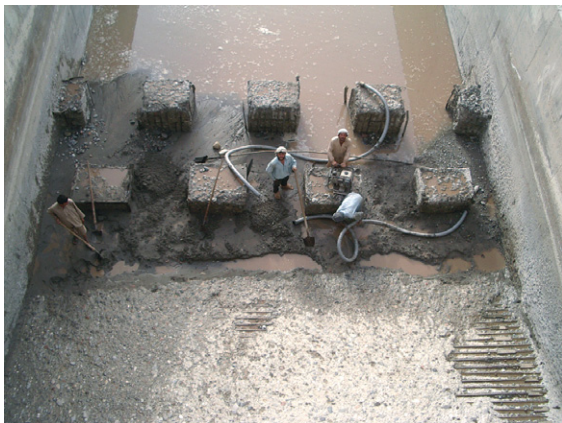
Figure 7 Erosion of concrete by flowing water.
