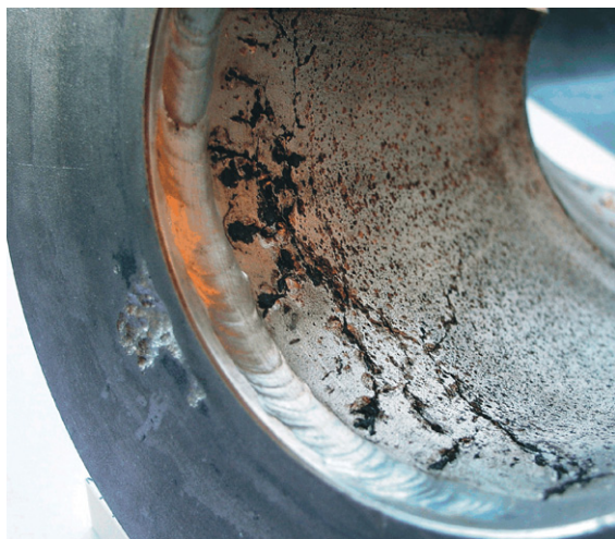
Figure 11 SCC, crevice corrosion, and pitting corrosion on a stainless steel pipe, after service in a very aggressive environment consisting of high amounts of chlorides, water, and oxygen in combination with high temperatures under evaporative conditions. Photo: Outokumpu Stainless.
