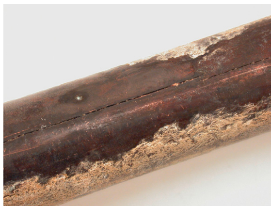
Figure 6 Photograph showing longitudinal stress corrosion cracking of a 15 mm diameter copper tube (EN 1057, R250, half-hard condition).
