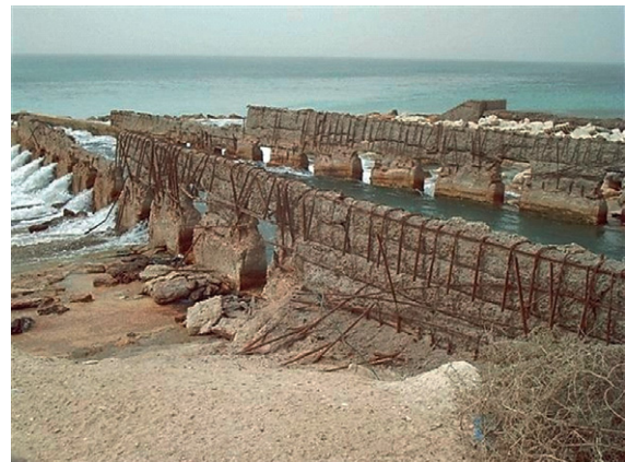
Figure 8 Exfoliation of a seawater outfall.
